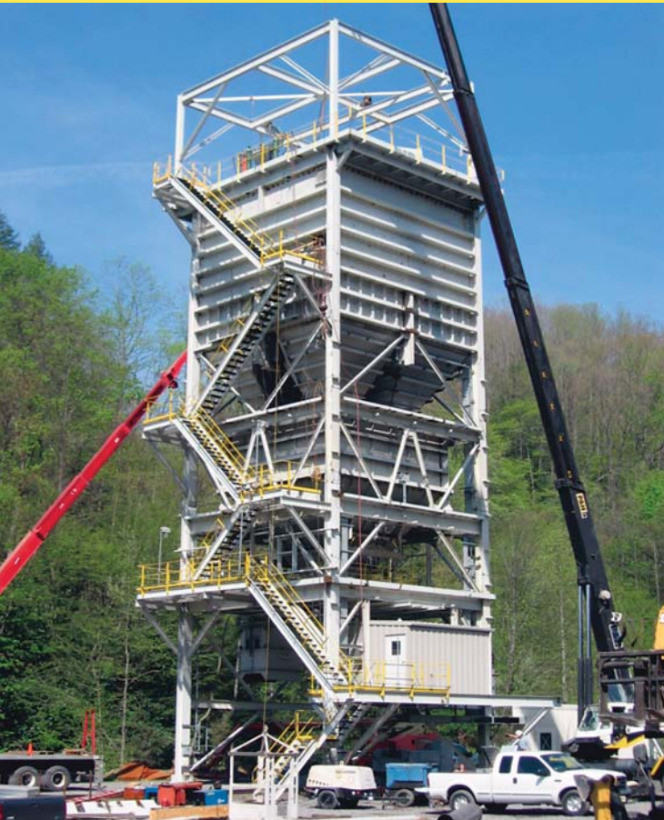
Unit train loadout with a 400 ton surge bin Wise County, Virginia • Completed April 2007
